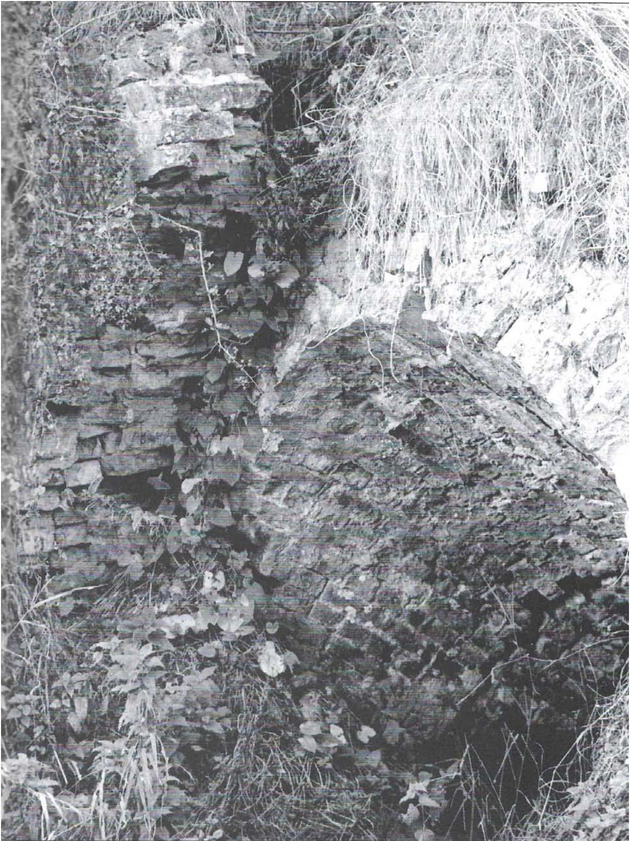
The collapsed brick headwall and the inclined outlet of the Alvingham mill tailrace siphon as it emerges from under the Louth Navigation. This siphon was abandoned when the lock gates were removed and the navigation water level lowered in 1941/42. From this time on, the tail race has discharged into the navigation, and not to the Lud as it did previously. (Photo: The author, November 1995).
