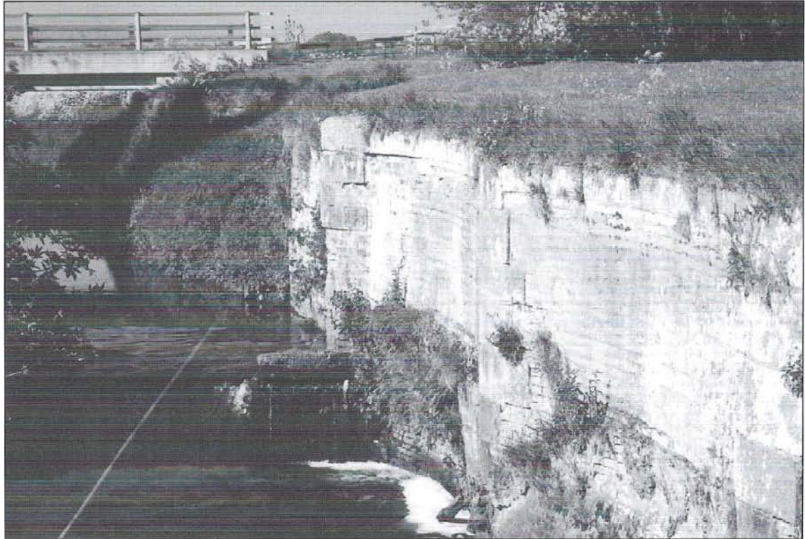
The north west wall of Alvingham lock chamber looking southwest towards the new concrete road bridge. (Photo: the author, 1999).
