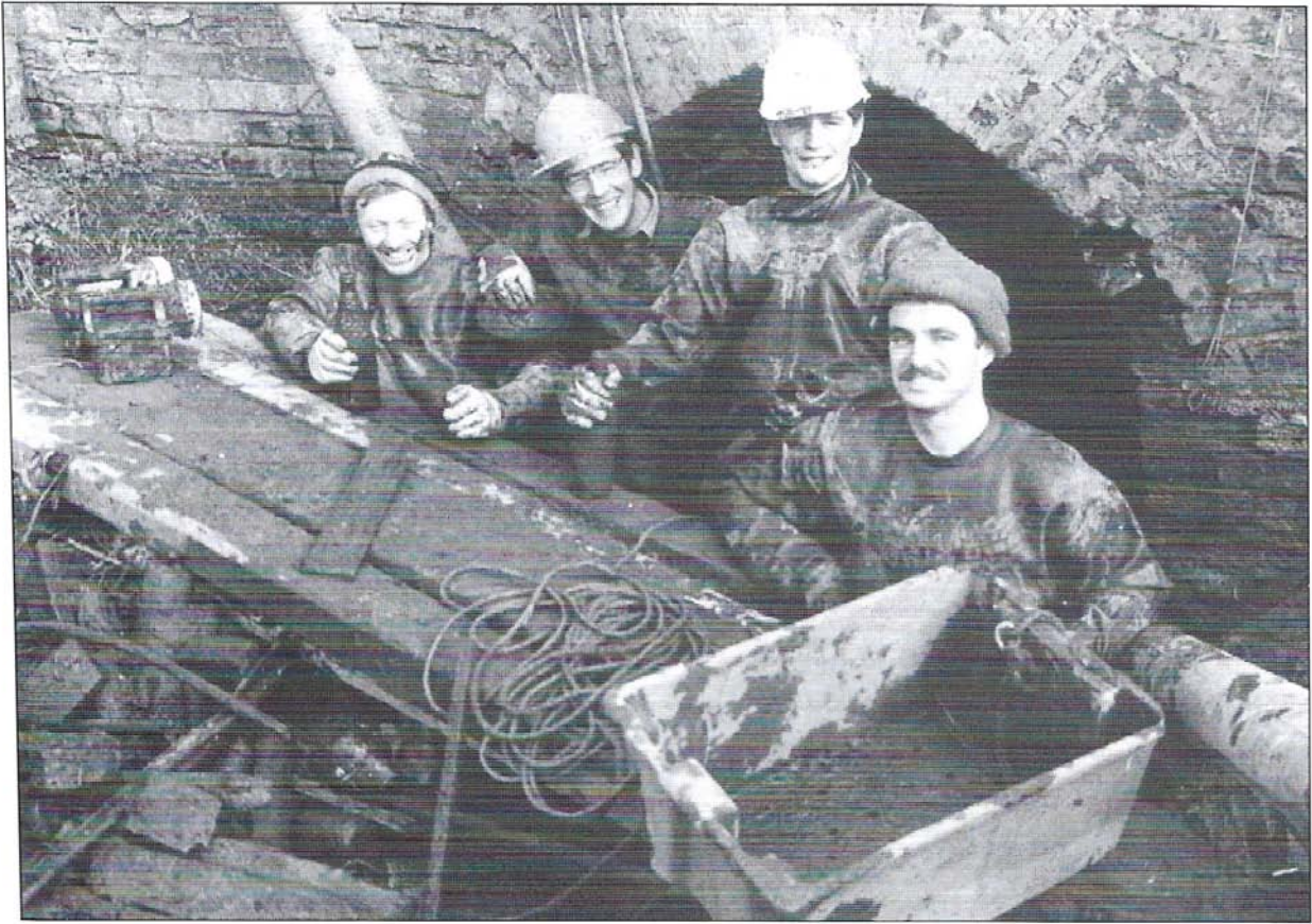
Workmen clearing out the 5ft. Diameter brick siphon which carries the millstream under Alvingham lock. (Photo: Grimsby Evening Telegraph 1981).
